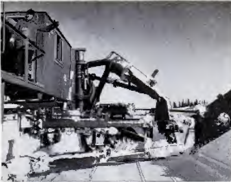
Huge machine used for spreading ballast along the tracks doubles in winter as railroad snowplow, cutting through 10-ft. drifts with steel "wings" that stretch out 25 feet on either side
